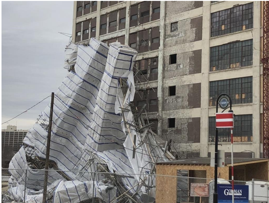
Collapse of scaffolding at the Amerock building
