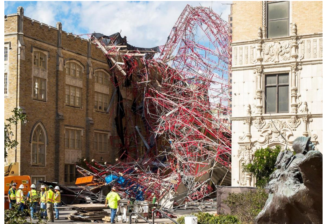
Scaffolding collapse in downtown San Antonio
